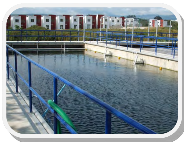
Tuxtla Gtz. Chps. 40 lps.
